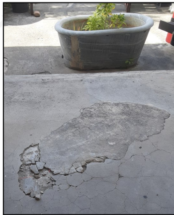
Scabs of cement plaster breaking up exposing limestone structure on platform and steps.
