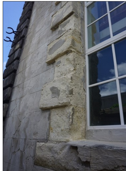
Deteriorating outside walls of the museum building
