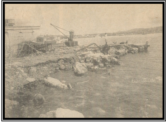
Bryson Wharf landing point for local and inter-island schooners was destroyed beyond recognition.
