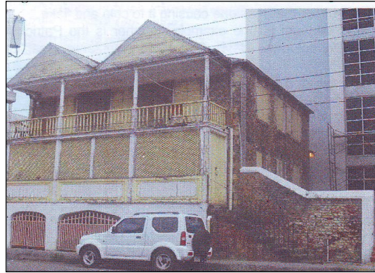
Once a dwelling, the 19th century residence above is constructed of bricks, limestone and wood. Over the years it has undergone several renovations that have altered its original features. Eventually it was used as offices, but is now empty and deteriorating from neglect.
